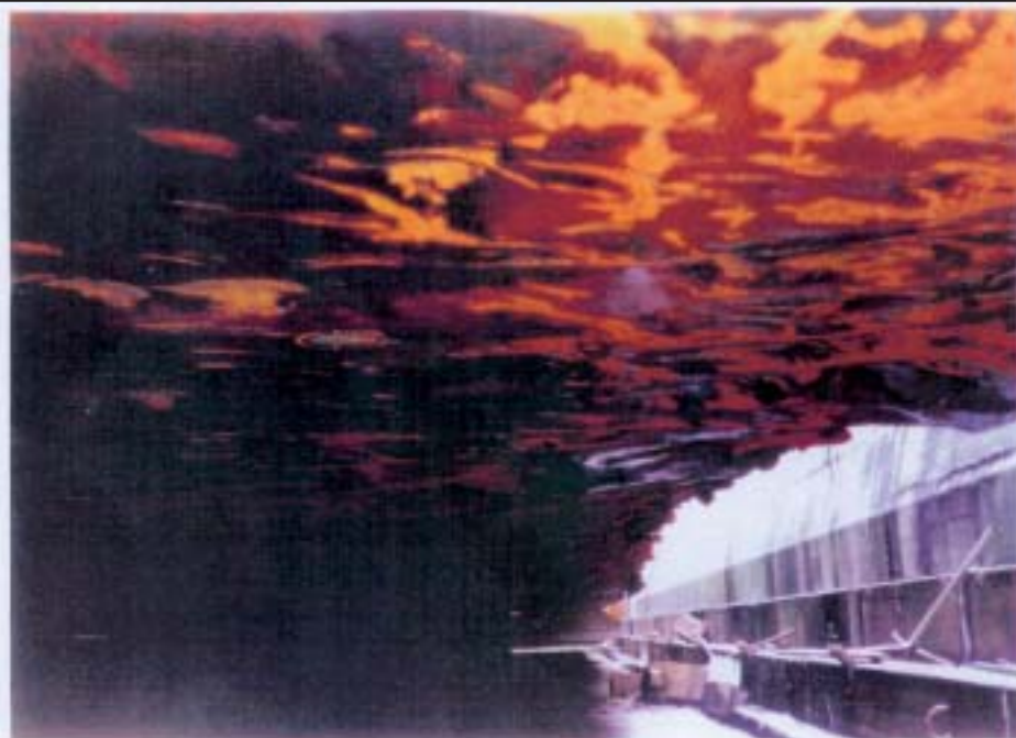
PHOTOGRAPH NO. 3 BOTTOM SHELL
