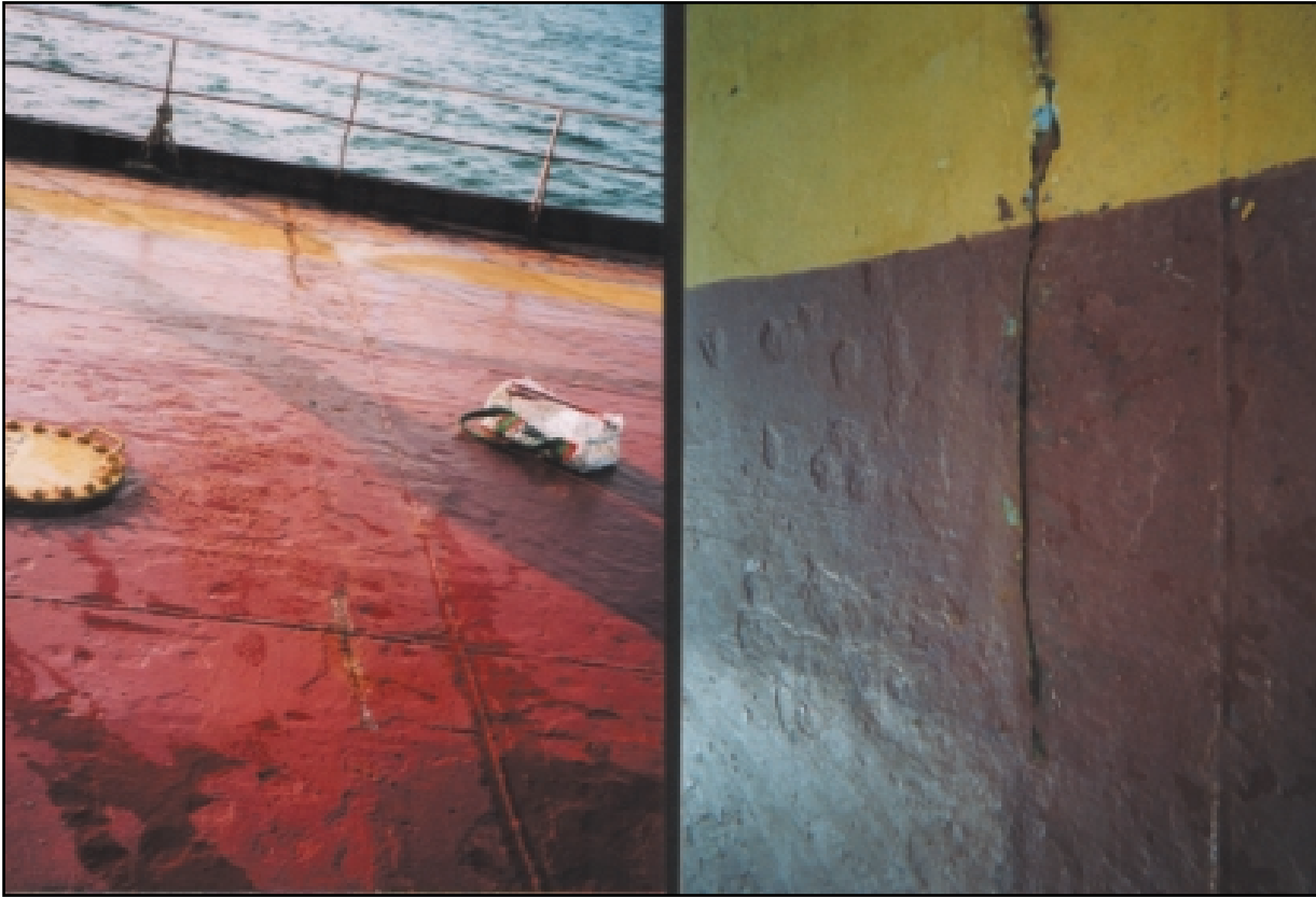
Figure 7.1.5 Double crack at frame 69 port side 1.6 m long at ship's side and 1.2 m long inboard in way of No. 2 WBT aft bulkhead with No. 3 COT
