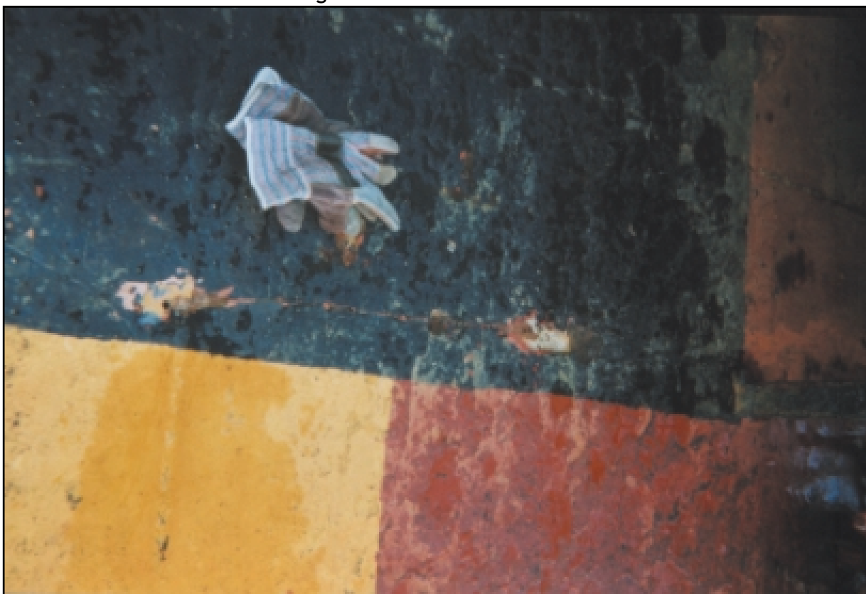
Figure 7.1.4 Deck at frame 59 port side showing same crack and general spot corrosion wastage of deck
