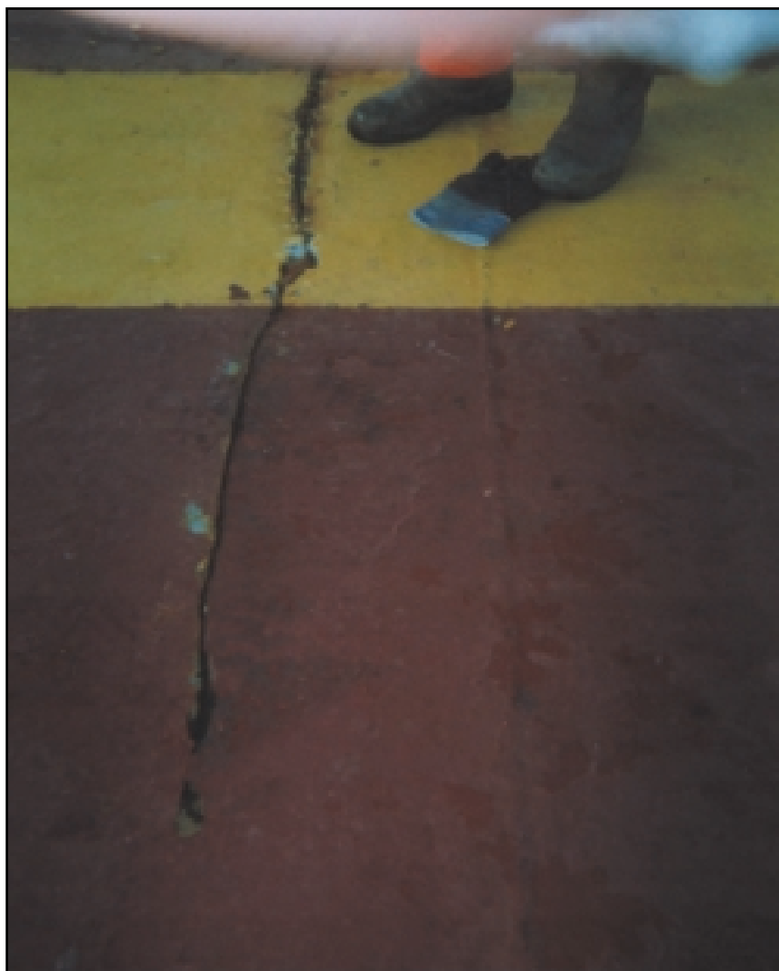
Figure 7.1.7 view of 1.6 m crack from above deck
