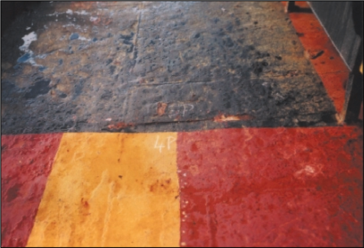
Figure 7.1.3 Crack at frame 59 port showing (top) cargo manifold save all and (bottom) to ship side length of crack approx. 0.65 m
