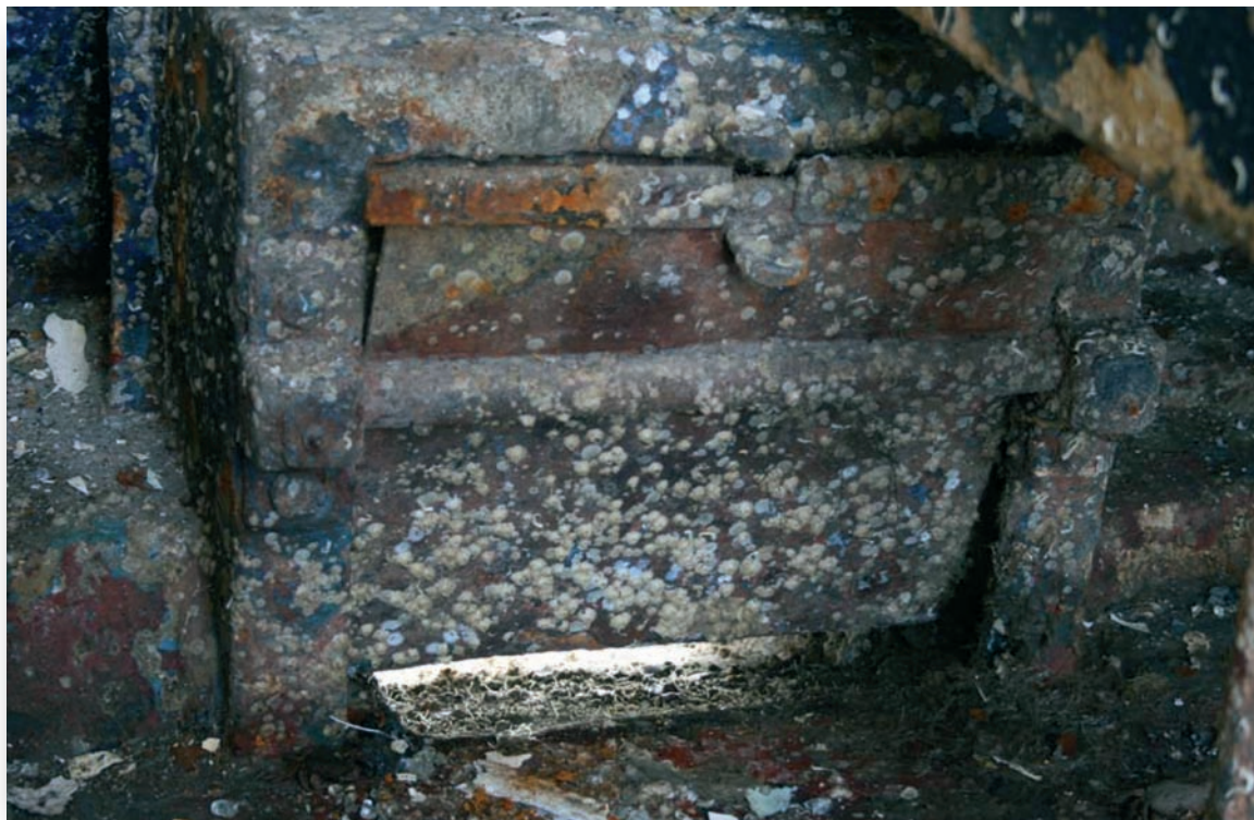
Photograph 8 - Freeing Port D (Port) viewed from inside (showing siezed hinged cover).
