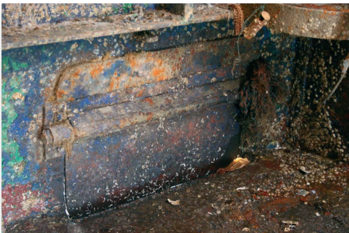
Photograph 5 - Freeing Port C (Port) viewed from inside (note 'small hole' just forward of freeing port).
