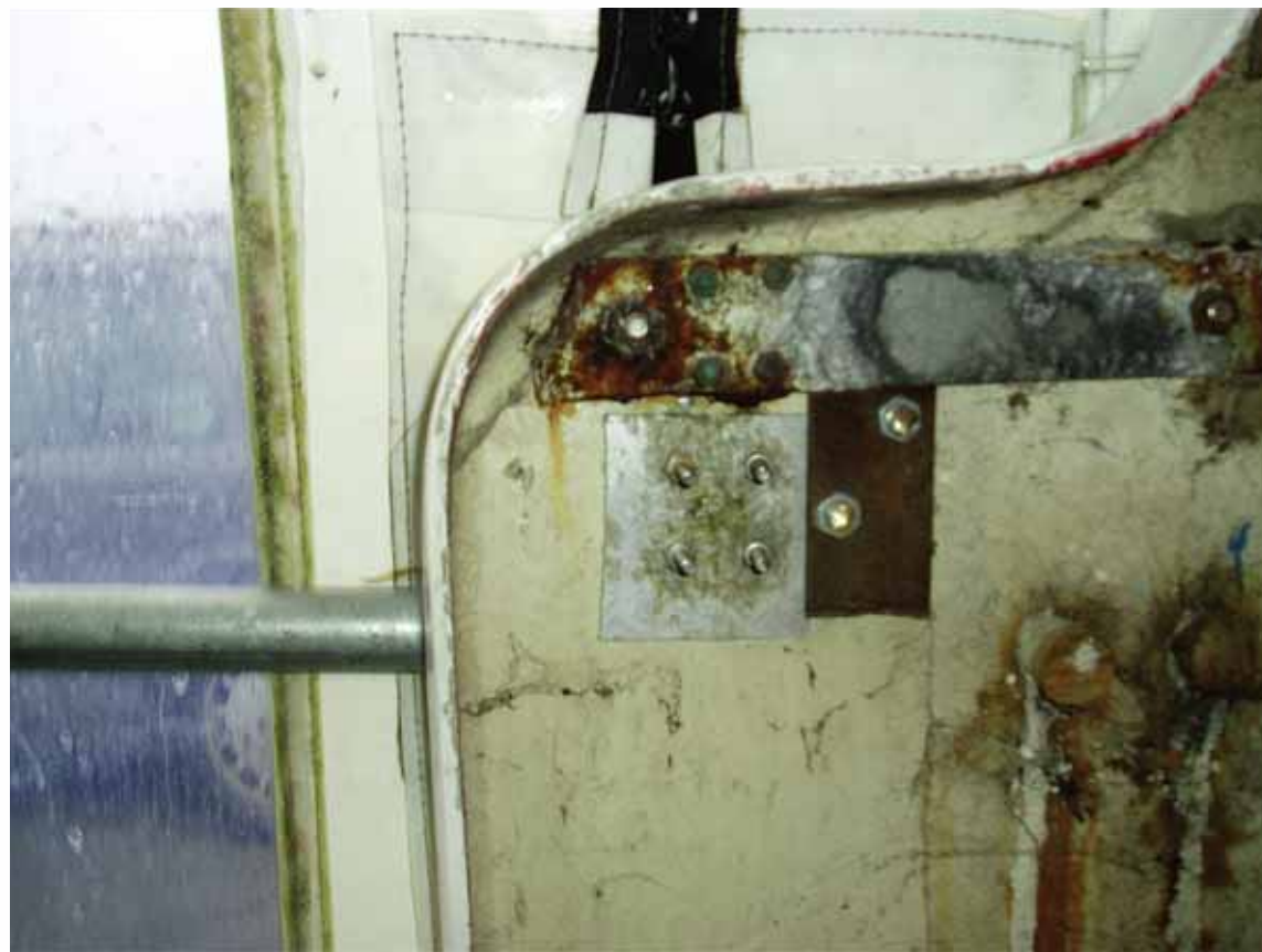
Appendix 9.5 View of inside of cabin structure showing backing plates for fixing to glass fibre.
