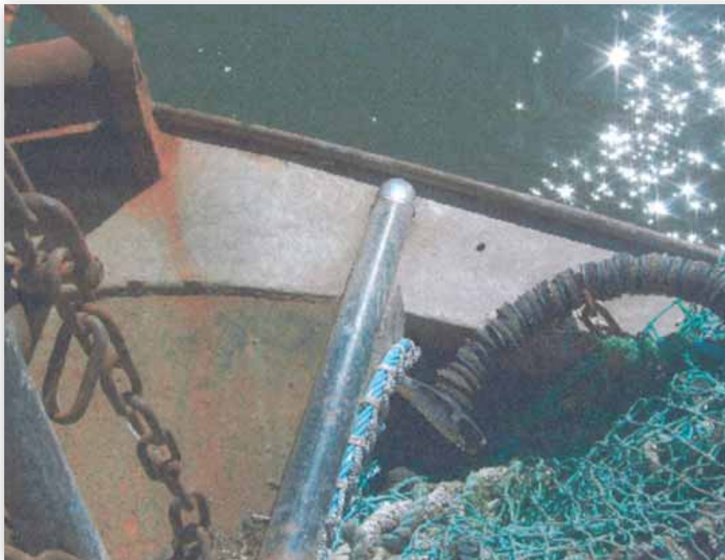
Photo 3 - View of the portside aft area of bulwark rail capping arrangements.
