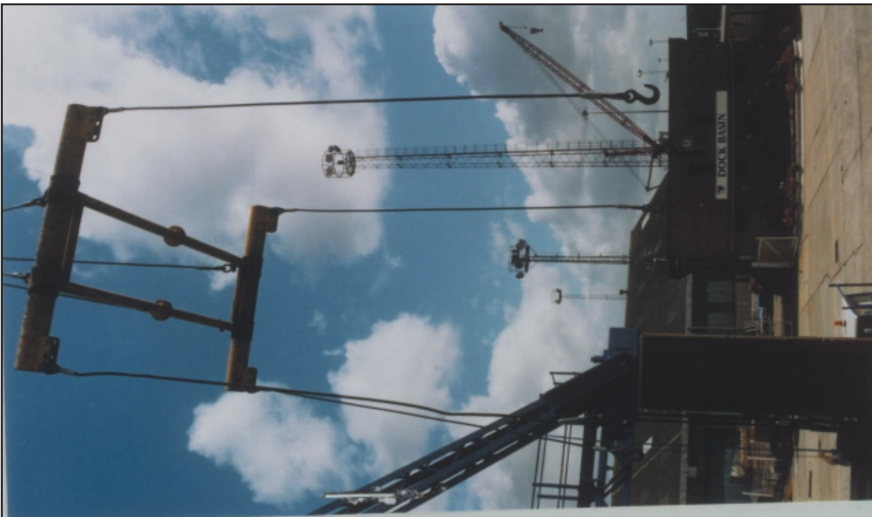
Photograph “c” shows a wire lift with wires hanging from a manual spreader frame with the hooks connected to the trailing ends.
