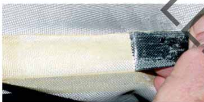
Adhesive in good condition - beige in colour FIGURE 4
