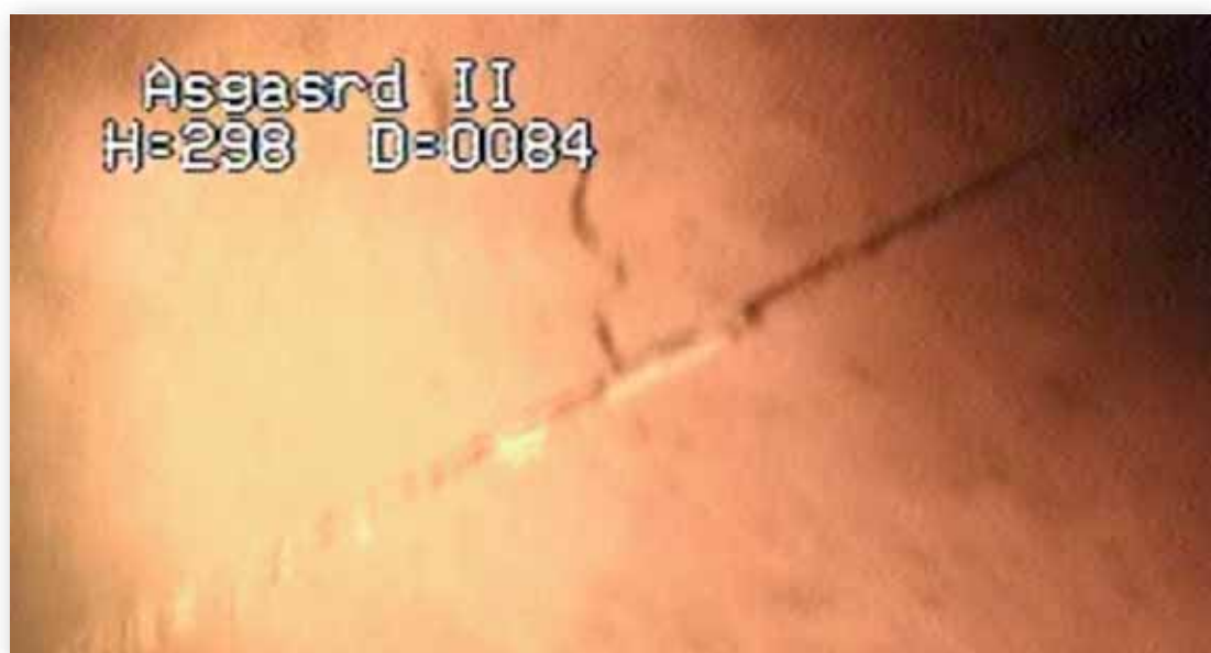
Photo 4 - Cracked Hull Plank (portside).
