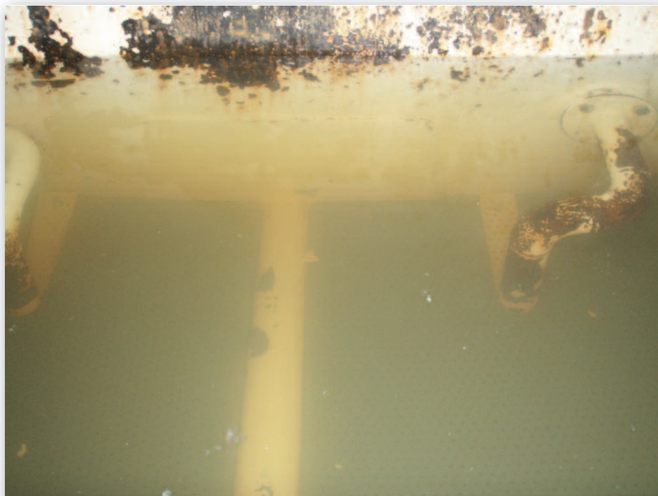
Pipework within tank.
