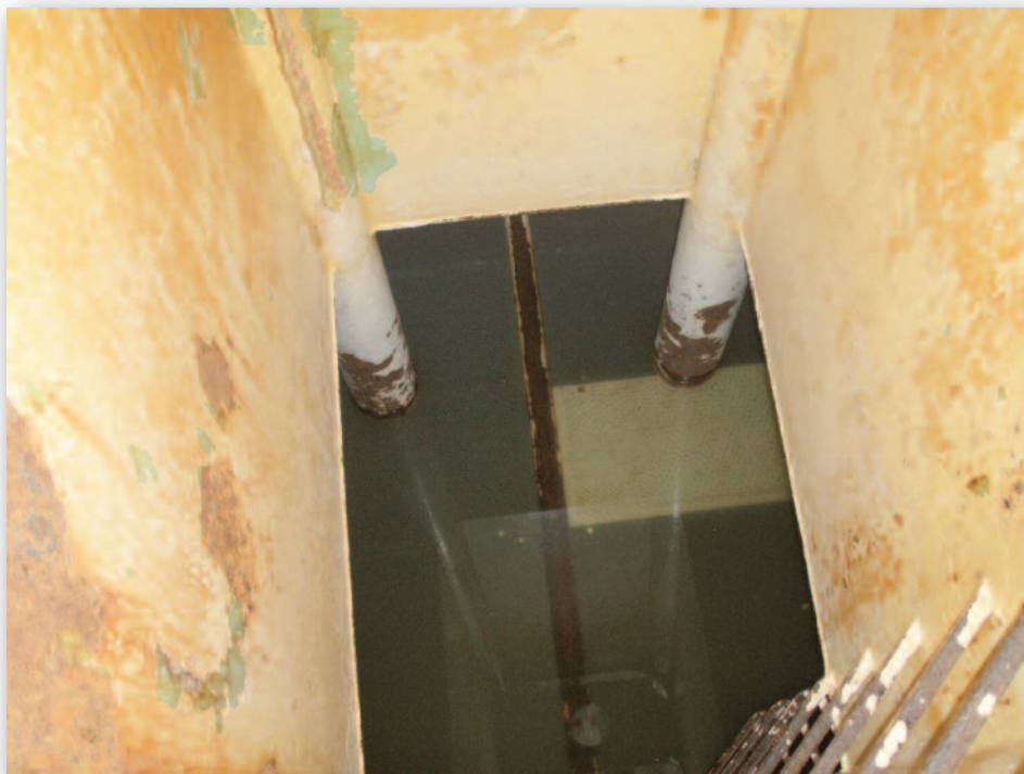
Vivier tank trunking.
