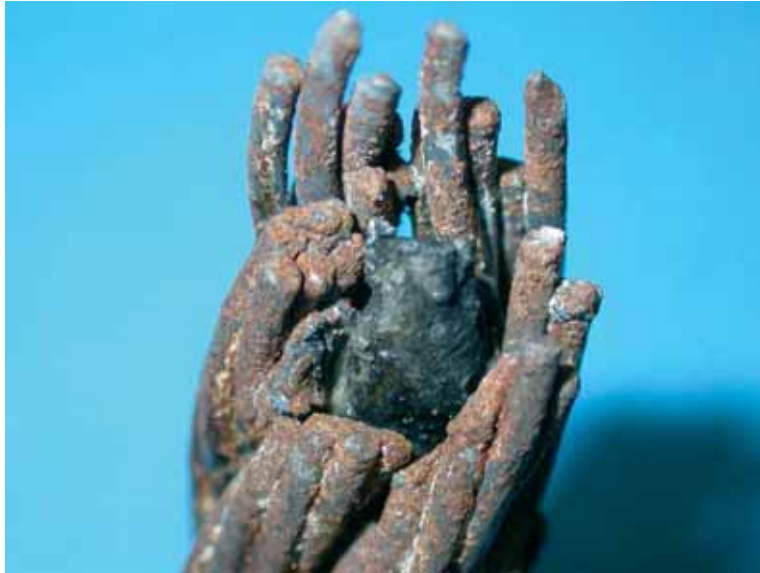
Figure 23: Port Side Fixed End sample, showing melting of strands, individual wires and the polymer core.
