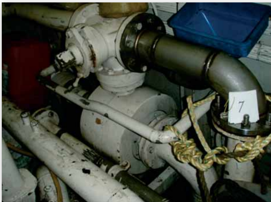
(e) IVER Pump (note stainless outlet pipe on bend).
