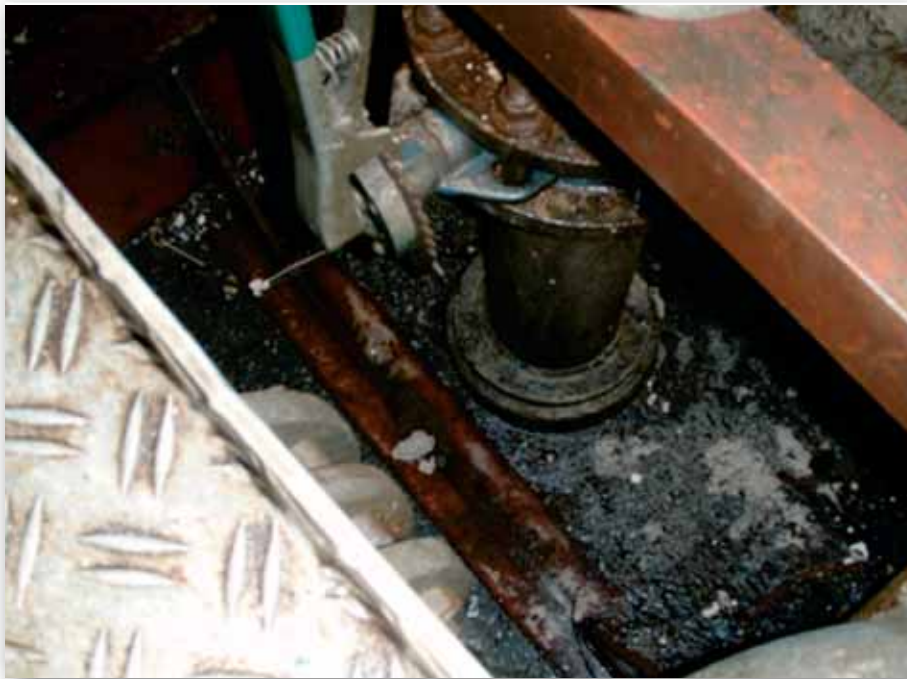
(c) The hydraulic oil cooling water inlet.
