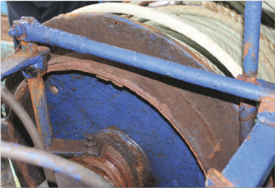
Photograph No. 9: Winch Break Band Note Excessive Corrosion. The Winch was being used in the Lifting Operations
