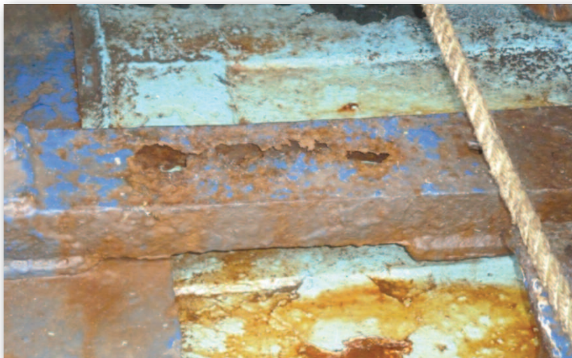
Photograph No. 12: Winch Corroded Foundations
