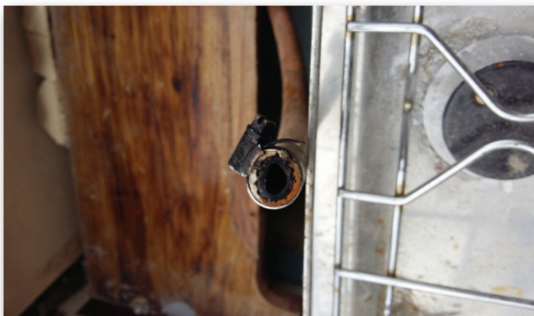
Photograph No.5 - Gas hose cooker end as found, charred and distorted.
