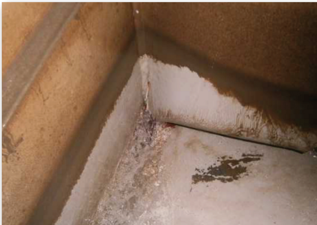
Photograph No. 3: Internal damage, distortion of internal frames.
