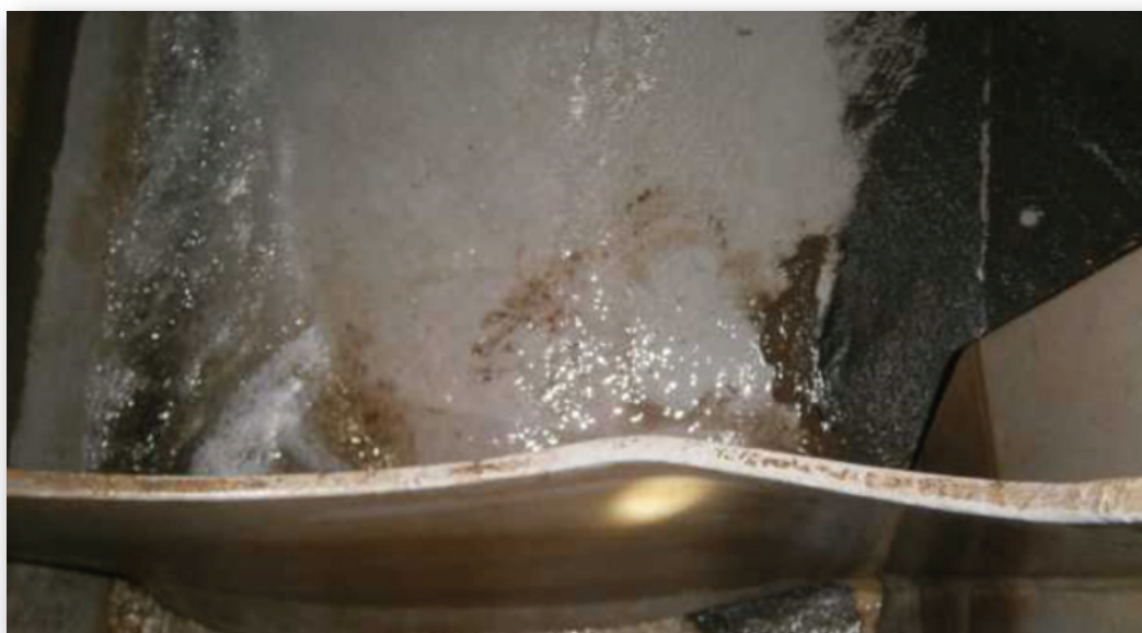
Photograph No. 4: Internal damage, distortion of internal frames.
