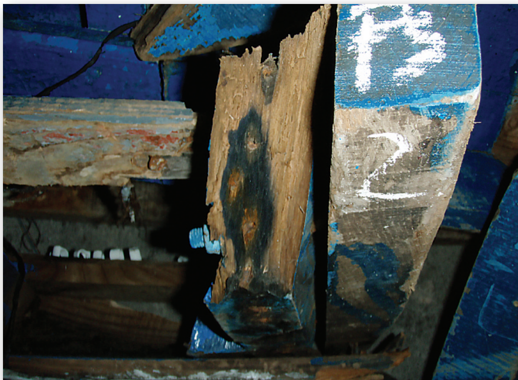
Photograph No. 3: Frame from port side, showing fresh break.
