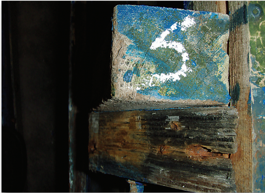
Photograph No. 5: Another frame from Starboard side, showing old break.
