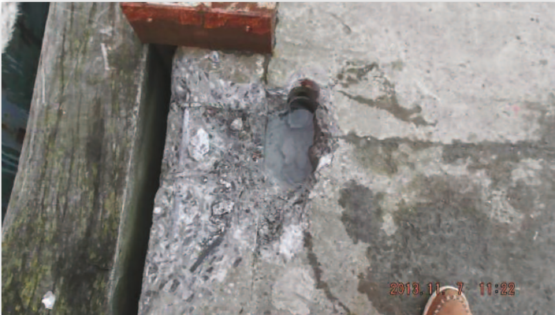
Photograph No. 7 - Hole in apron left by mooring ring, with cracks radiating out from bottom end
