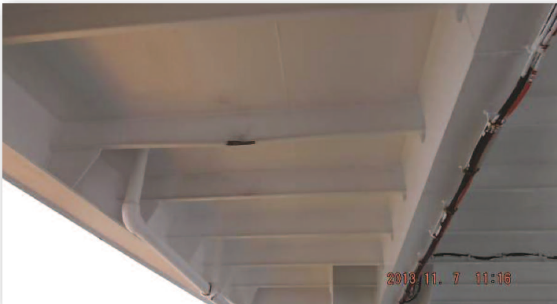
Photograph No. 6 - Damage to deck support beam, starboard side poop deck section
