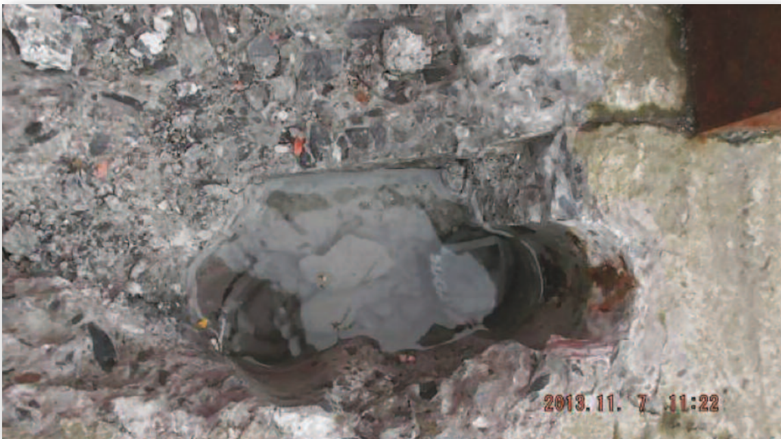
Photograph No. 8 - Looking down into hole, no anchoring points visible
