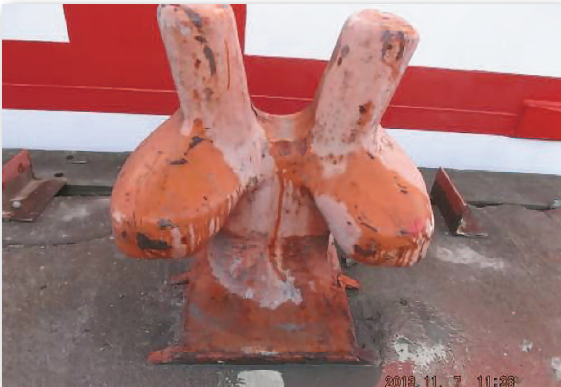
Photograph No. 10 - Stag horn bollard on quay - type of mooring that should have been used
