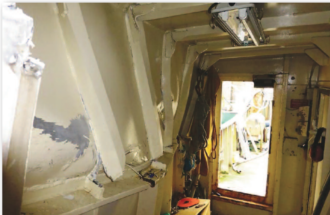
Photograph No. 12 - Damage to “MFV Ocean Dawn”
