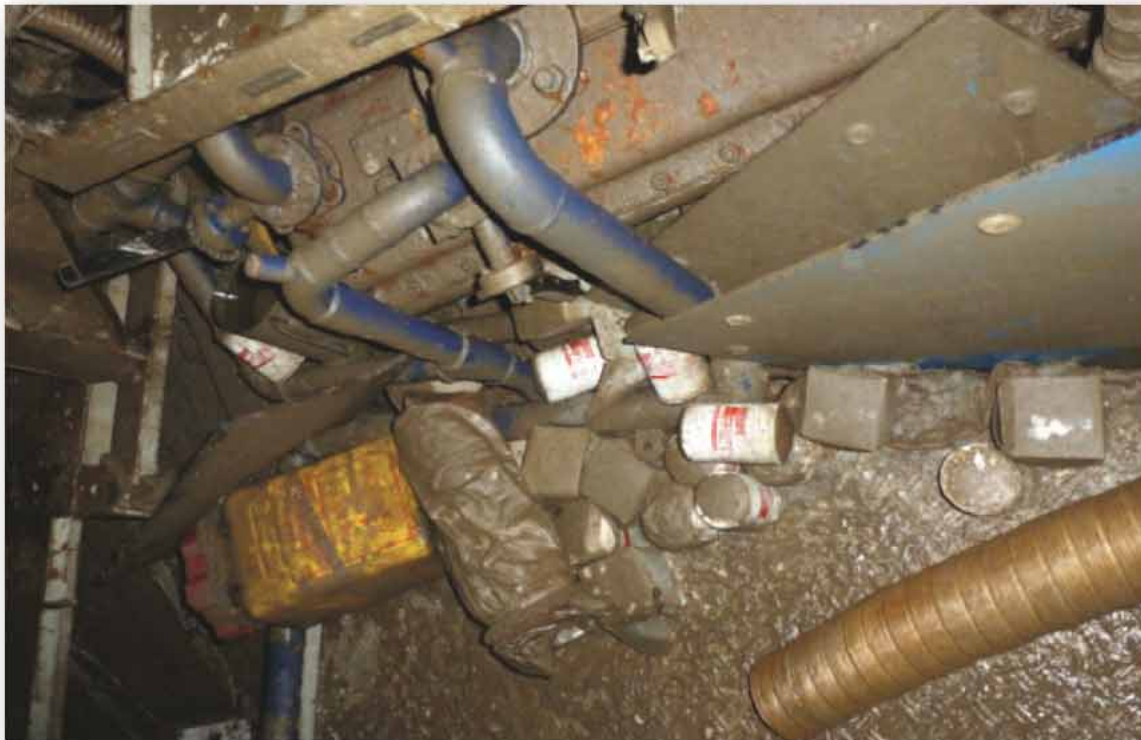
Photograph No.18 - Fuel filters found lying in engine room
