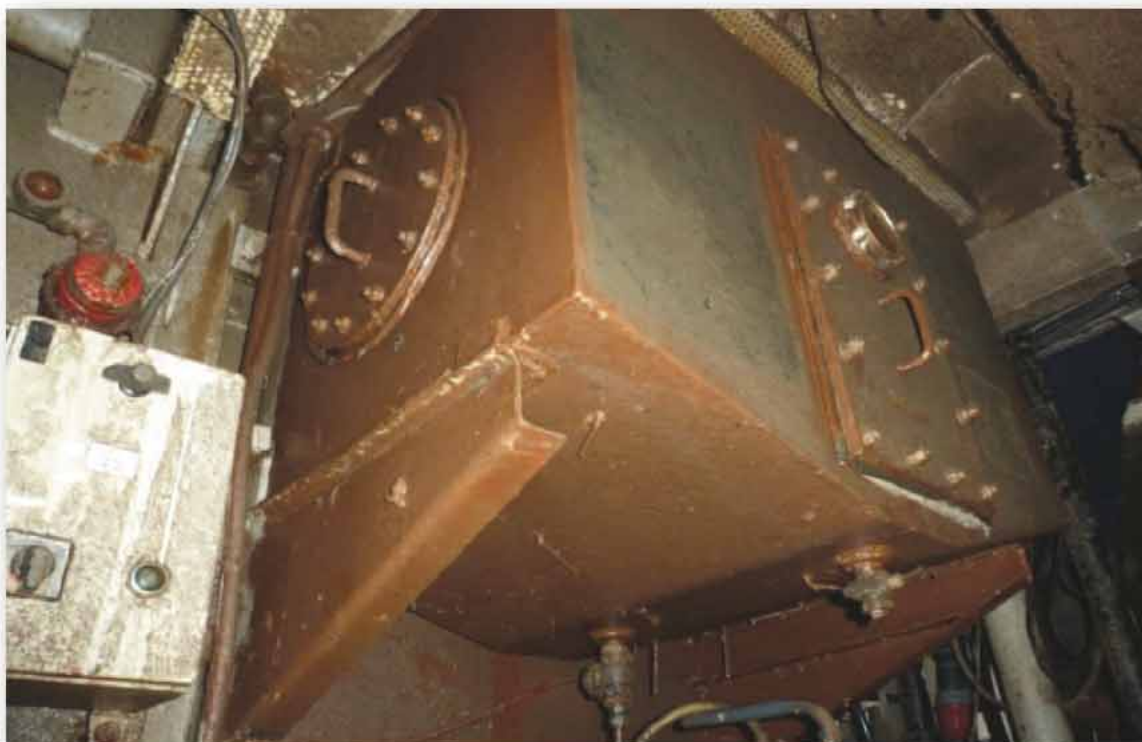
Photograph No.16 - Fuel oil daily service tank full of seawater as expected
