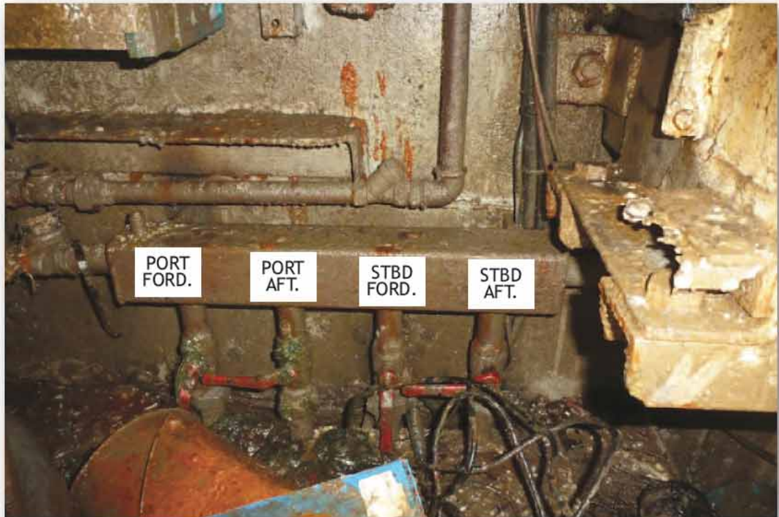
Fuel Suction Valves in Engine Room Port Forward and Starboard Forward Found Open
